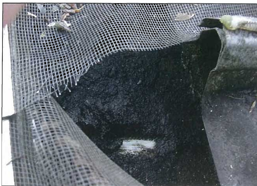
Figure 4-8: Mobilisation of organic matter into a gutter leading to putrefication of tank water
